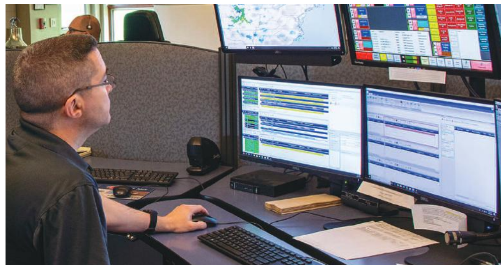
Greene County 911 Center systems administrator Neil Kellegher on duty in the deeply emotional and highly technological world of telecommunicating.
