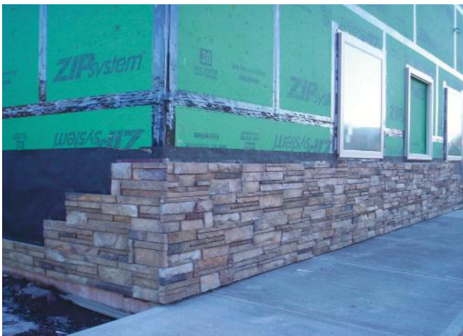
Stone veneer siding has started to be applied to the exterior of the new ambulance center in the town of Windham.
