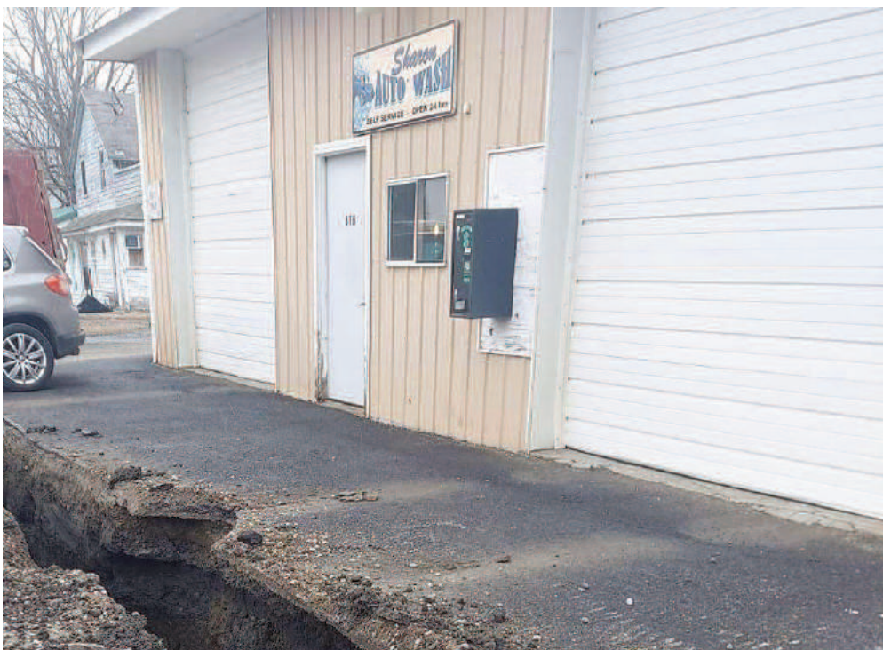
Sharon Springs Water & Sewer Project at work in front of the Sharon Auto Wash.
