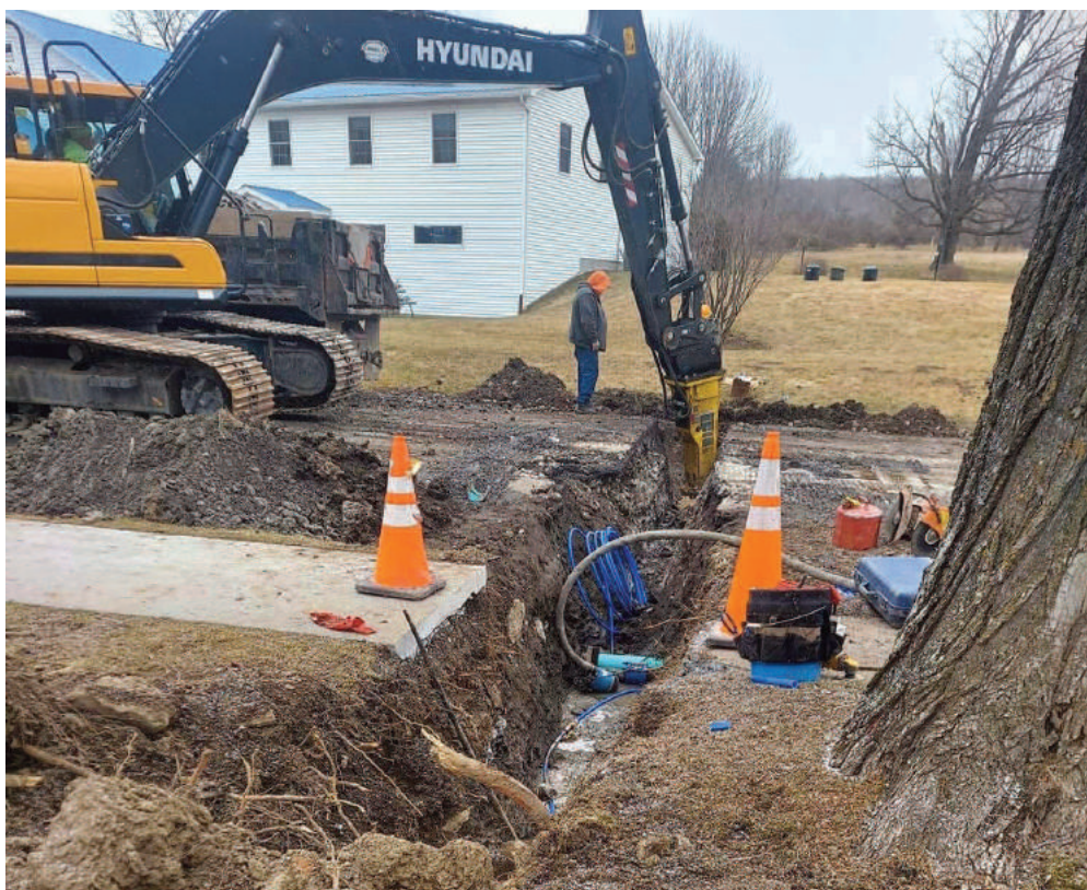
Large equipment rip up ground for Water & Sewer Project on Chestnut Street in the Village of Sharon Springs.
