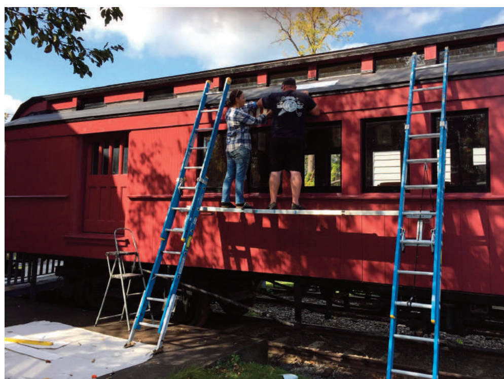
The painting work on the Mill Building, the Passenger Car, the Weigh Station and the Palatine House was done by DeGross Painting, and the letters were made for us by True American Signs of Cobleskill.
