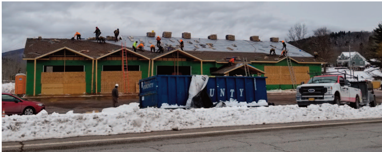
A platoon of roofers swarmed to the new ambulance building in Windham, readying the project for indoor finishing touches.
