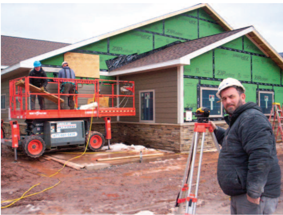
Terry Goyer, job superintendent from Plank Construction Services, checks the band boards, ensuring exterior siding of the new ambulance center in Windham is on the level.
