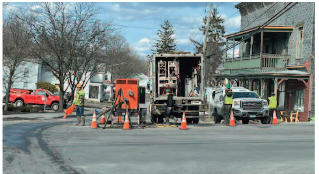
Repair crews working on a burst pipe under Main Street (3/29) in the Village of Sharon Springs leaving the Post Office and Bank without water all day.
