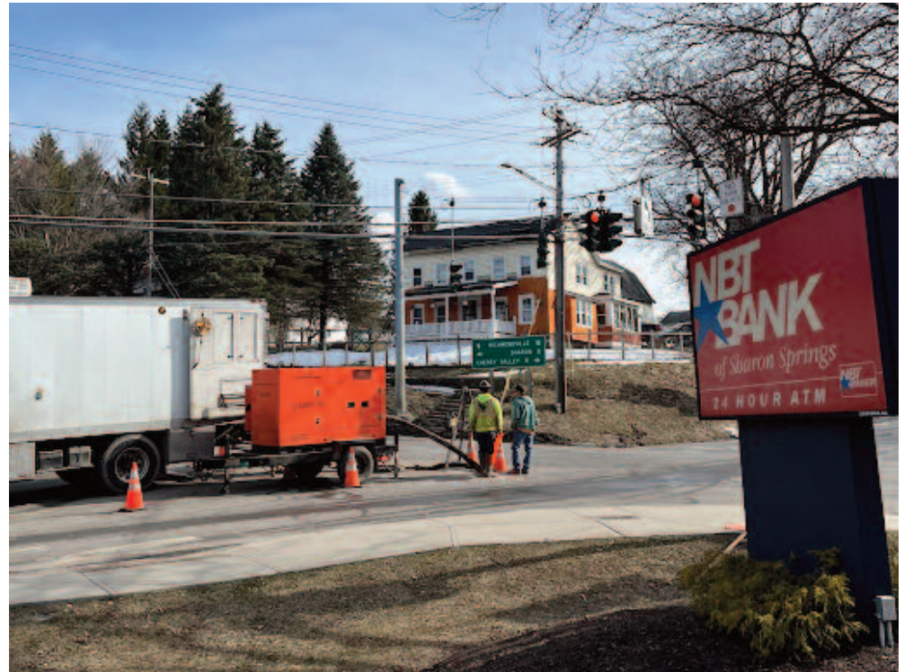
The Village of Sharon Springs Superintendent of Public Works Vladimir Jones was seen speaking with the repair crew at the busy intersection of Route 10 & Route 20 on Wednesday afternoon (3/29)
