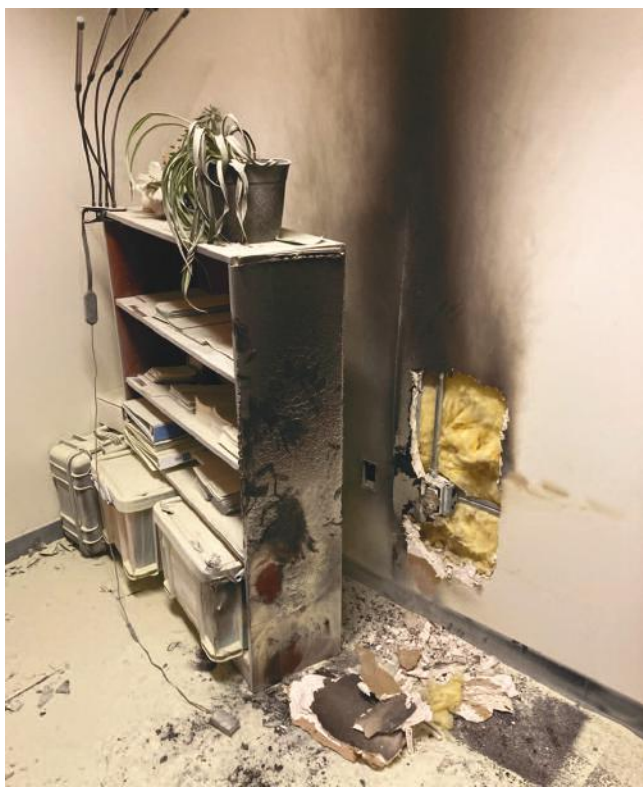
A fire in the Public Health Department at the Greene County Office Building in Catskill was fortunately short-lived.
